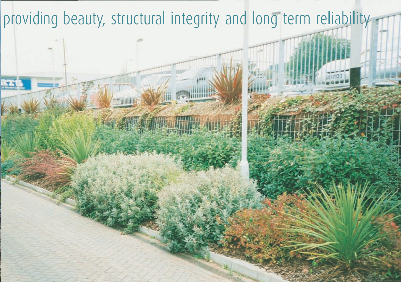
Vegetated faces can offer significant savings over more traditional forms of construction.
